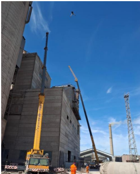
Support equipment for new raw mill 5
